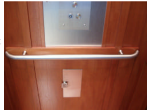
Handrail in Stainless Steel
